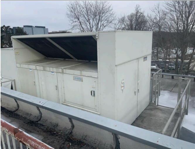
13 - ROOFTOP PACKAGED UNIT
