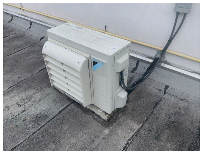
12 - DUCTLESS SPLIT SYSTEM
