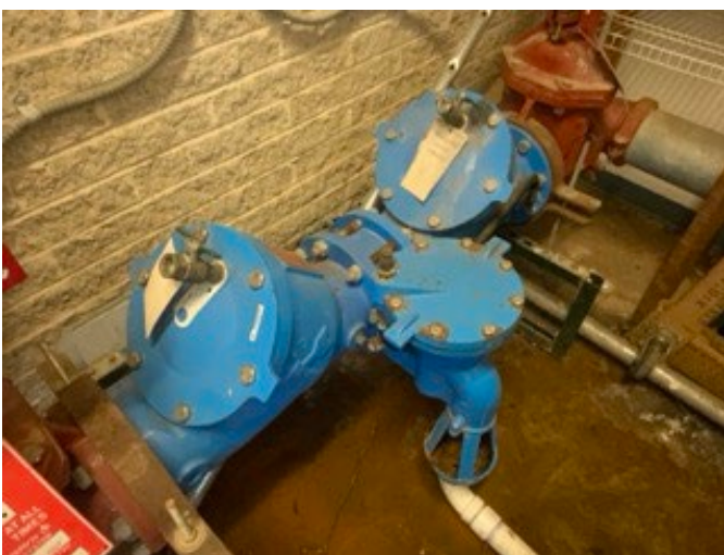
17 - SPRINKLER BACKFLOW PREVENTER
